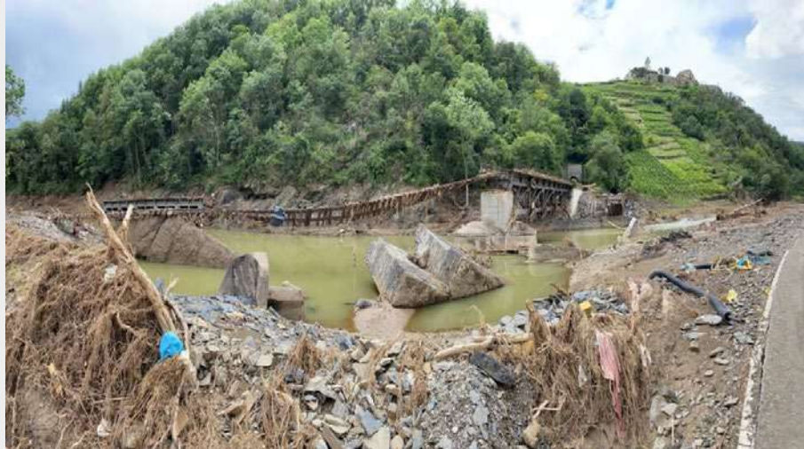
Figure 9: Flood in the Ahr valley, DB InfraGO AG, 2021
