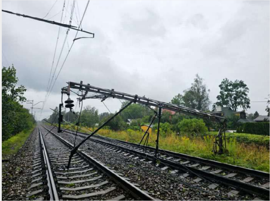
Figure 11: Storm damage in Latvia, Latvijas dzelzceļš, 2024
