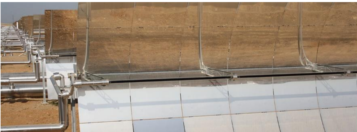
Figure 4: Africana Energía - Parabolic trough collectors
