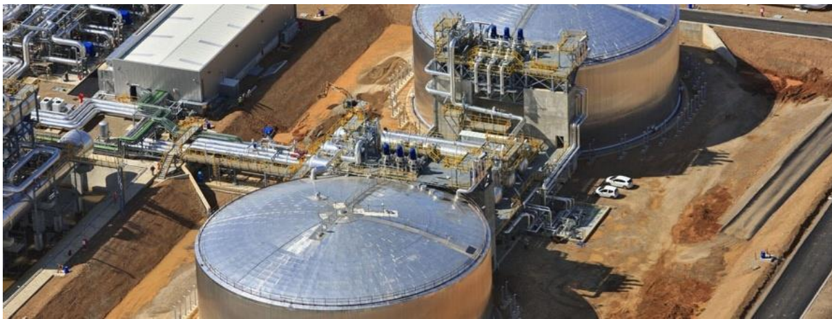
Figure 3: Africana Energía - Molten salts storage tanks
