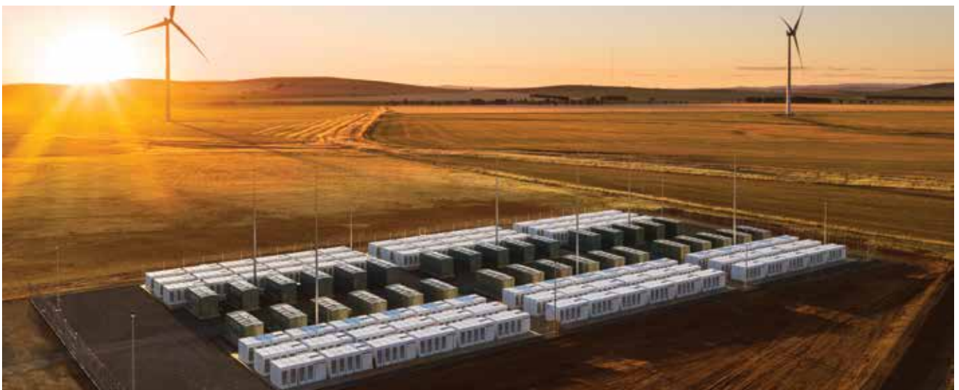
Figure 43: Hornsdale Power Reserve in South Australia
