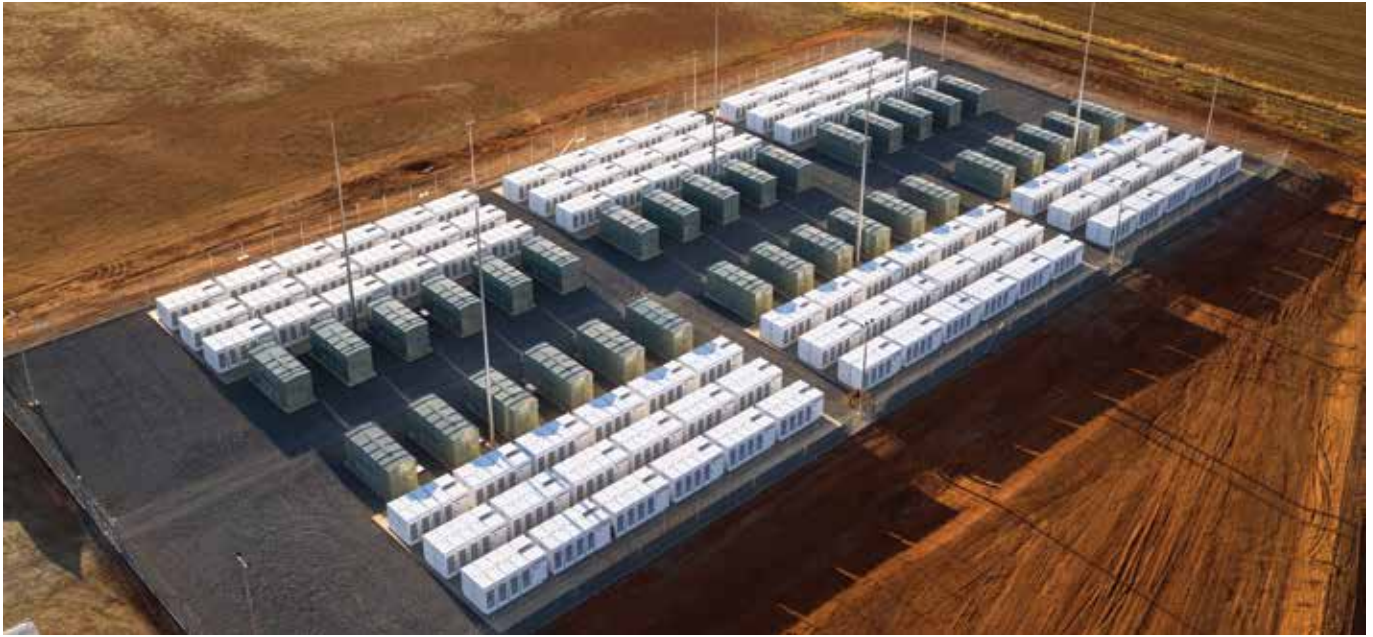
Figure 32: Hornsdale power reserve project in South Australia
